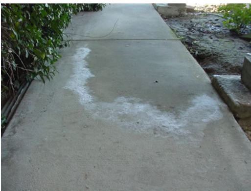
Figure 64: a case of efflorescence on a concrete pavement
