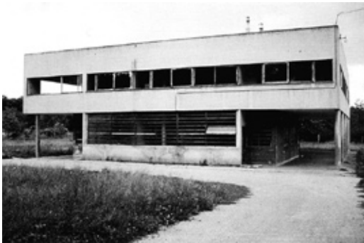
Figure 1 Villa Savoye 1929-1931 (Le Corbusier): state before restoration (1963-1997). Source: “On Weathering, the Life of Buildings in Time”
