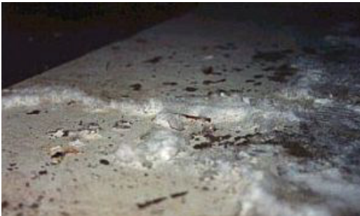
Figure 66: a close view on efflorescence Source: www.cuttingedgecurbing.com
