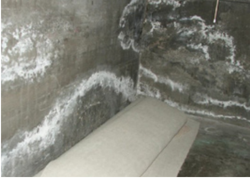
Figure 65: a case of indoor efflorescence Source: www.activerain.com
